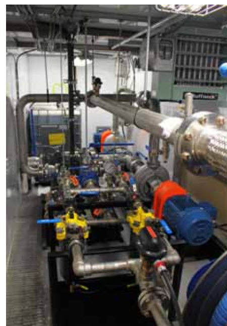
PUMPING AND FILTRATION
