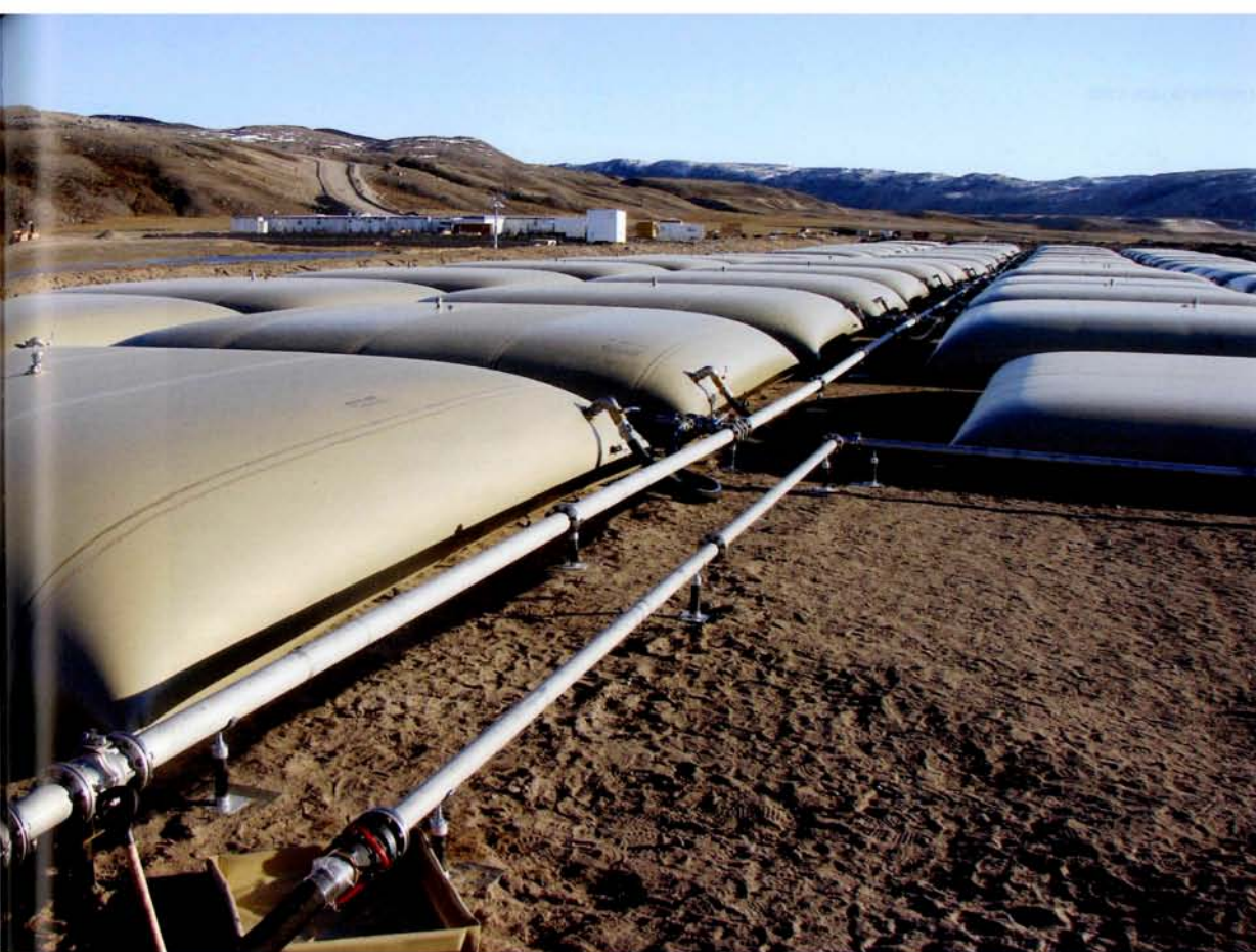
Ninety Arctic King tanks comprising a fuel tank farm for the Baffinland Iron Ore Mine.
