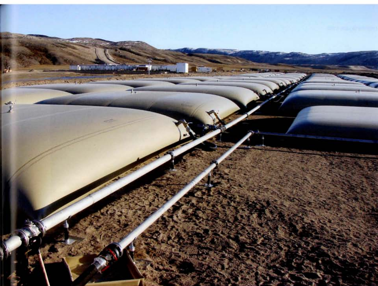
Ninety Arctic King tanks comprising a fuel tank farm for the Baffinland Iron Ore Mine.
